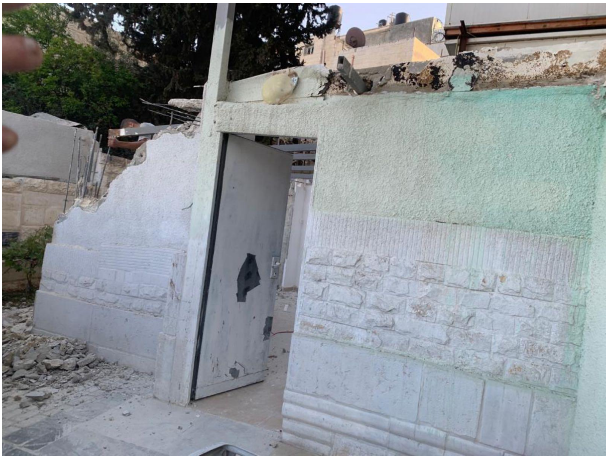
Demolished house, Sur Bahir, East Jerusalem, 18 April 2023
